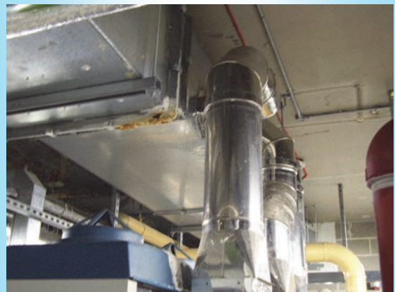
Chimneys and flues under corrosion testing
